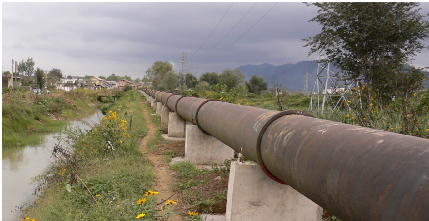
❖ Ductile Cast Iron water transmission line with a diameter of 800 mm
